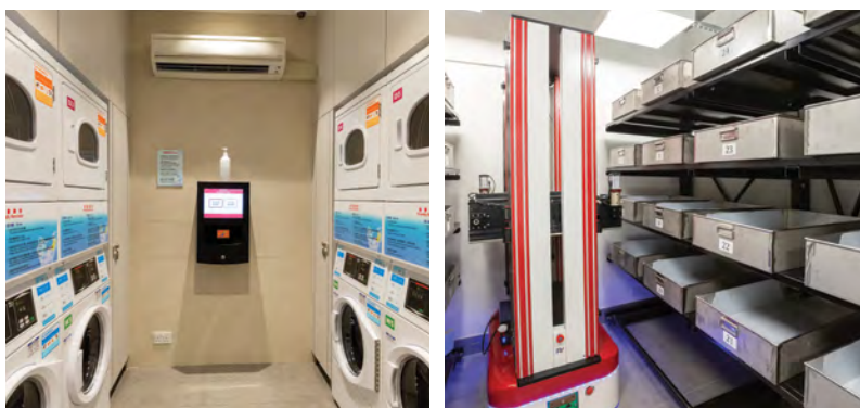
Smart communal facilities including eLaundry (left) and eStorage (right) are provided in eResidence.
