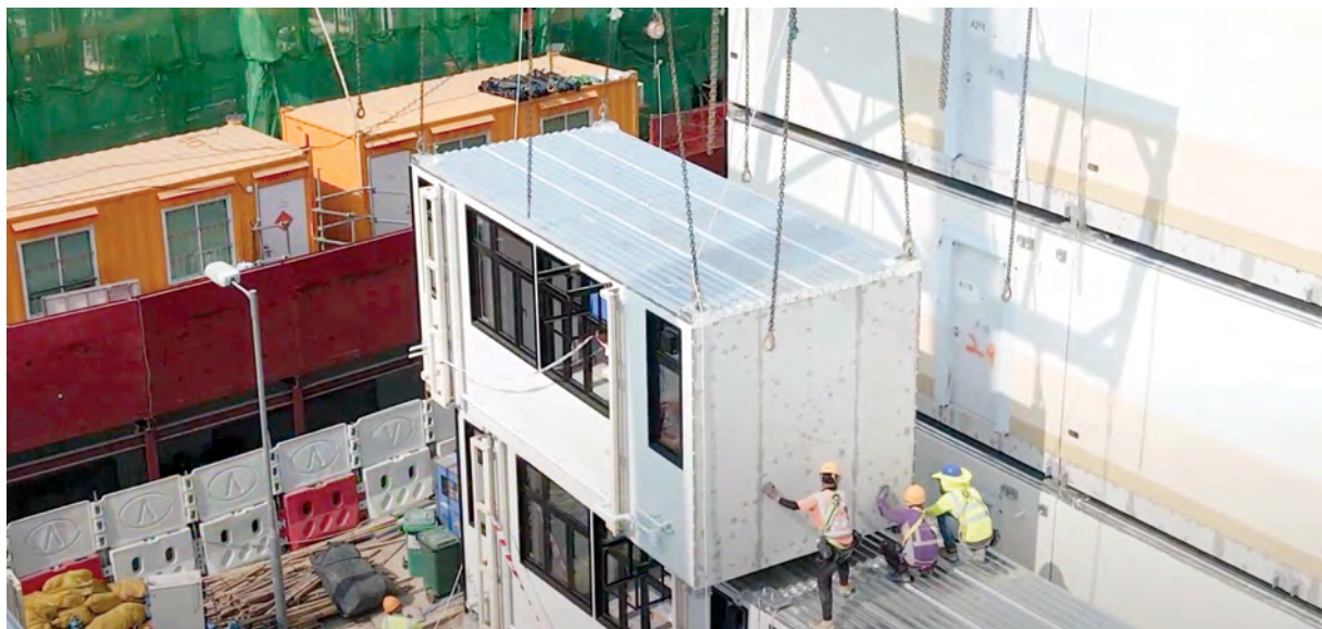
URA adopts Modular Integrated Construction (MiC) for the transitional housing project at Hung Shui Kiu for its sustainability benefits.
