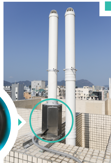
Installing the UV-C VentGuard on the rooftop ventilation pipe of rehousing block at Soy Street.
