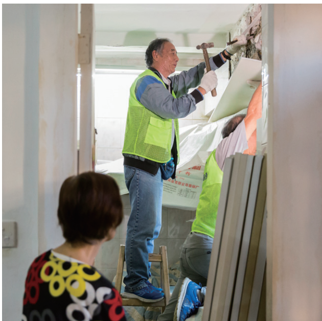
蔣師傅協助維修有石屎剝落的天花。 Master Chiang helps fix the ceiling to prevent concrete from spalling.
