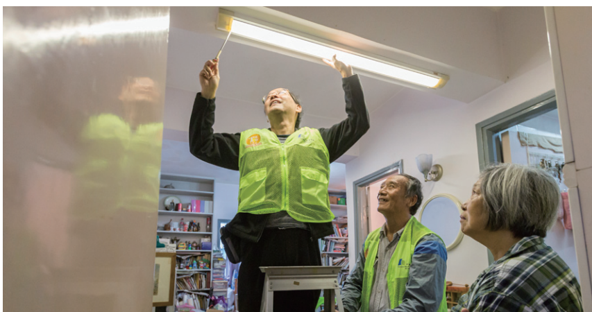
師傅義務協助獨居的周女士維修光管。 Volunteer repairmen help a single elderly Ms Chow to mend her lighting.
