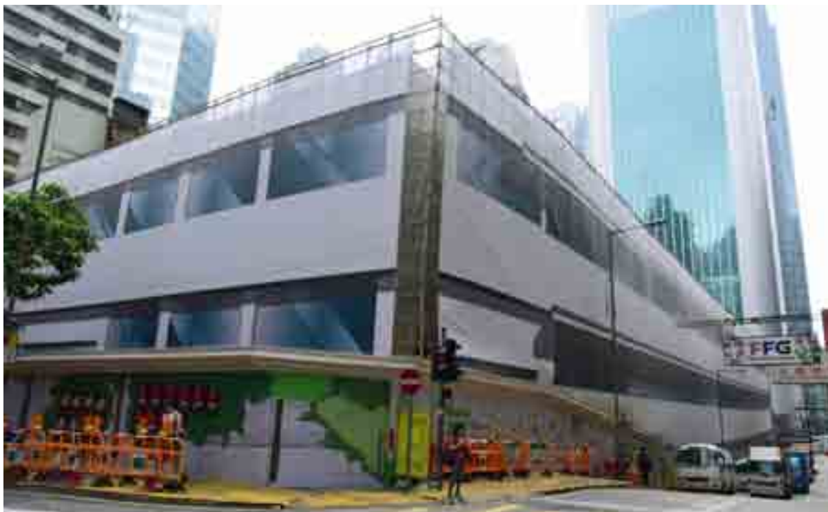
Central Market is now at advance works stage, mainly working at the areas near Queen's Road Central, which will become a new entrance plaza as part of the public open space.
