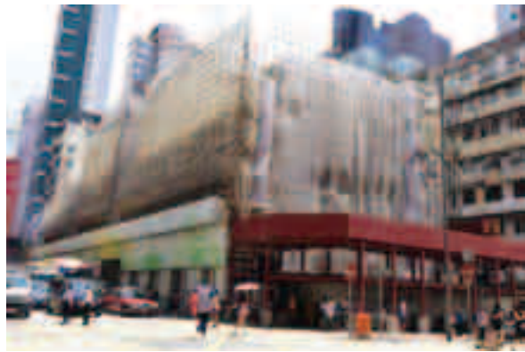
Superstructure works of Shanghai Street/Argyle Street preservation project is now in progress.
