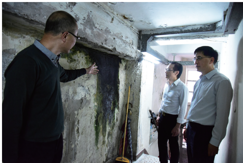
Visiting the Oak Street/Ivy Street project on the day of project launch and inspecting the varied and poor building condition with URA staff members.
