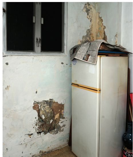
■ Poor building condition at the project site.
