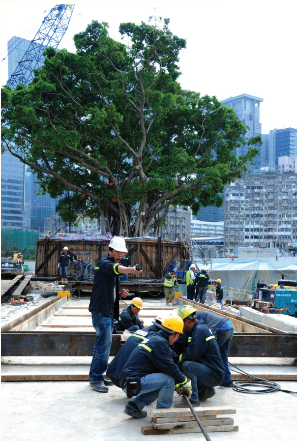
The first banyan tree is transplanted in the Kwun Tong Town Centre project.
