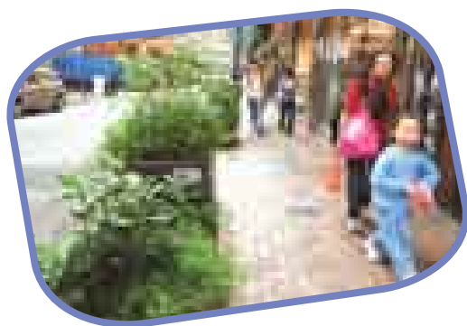
New paving and street planting in Tai Tsun Street, Tai Kok Tsui.
