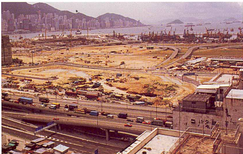
政府撥給房屋協會三個地盤，其一位於西九龍填海區，建成的樓宇將提供1,300個安置單位。 West Kowloon Reclamation, one of three sites granted by the Government to the Housing Society for the construction of 1,300 rehousing units.
