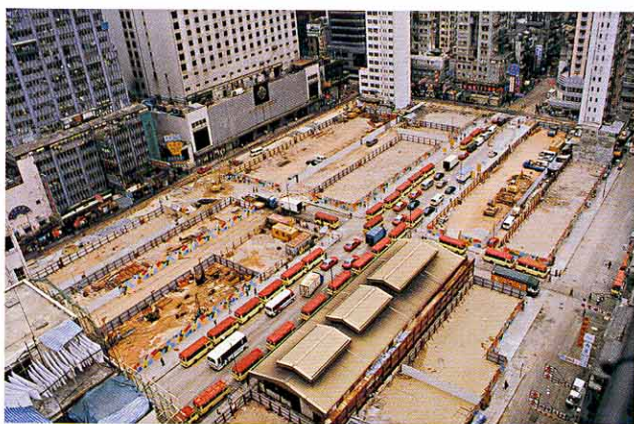
亞皆老街/上海街重建計劃的拆卸工程經已完成。 Demolition of the Argyle Street/Shanghai Street project site was completed.
